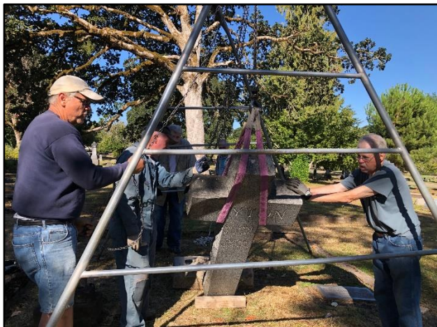
Left to right: Jeff Hilts, Dale Palmquist, and Mark Fields use straps and hoist to lift a leaning Payton cross, set it aside and build a stronger foundation. Gloria Hilts photo Aug. 24, 2020.
