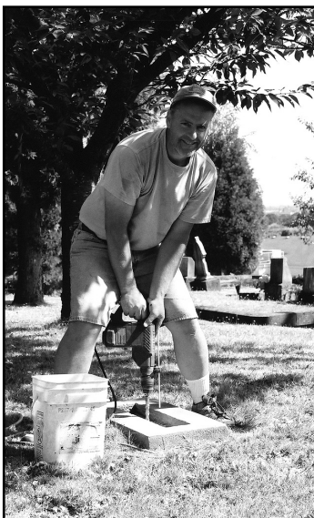
Last August, Jeff Hilts, proprietor of a Salem-based marker setting service, helped the Friends raise and reset the sinking headstone of Harvey Gordon. Hilts drilled and cleared the base keyway for added depth.
