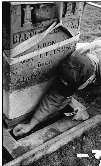
Dale Palmquist gave the Harvey Gordon headstone base a final check before mortaring its keyway newly cleared to a depth of four inches. The extra depth was appropriate for the height and weight of the stone.
